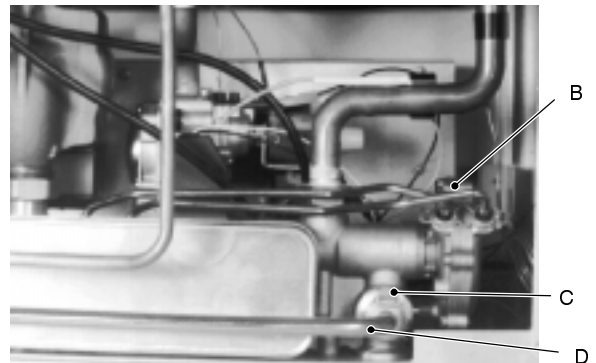
fig. 70 (rear view of the boiler)
