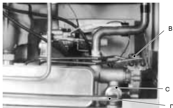
fig. 69 (rear view of the boiler)
